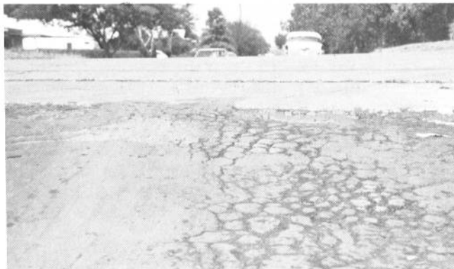
Loss of cover aggregate.
