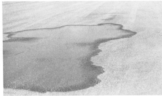
Water delineates depressed area.
